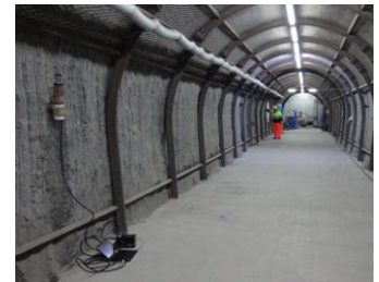
Buried data transmission underground
