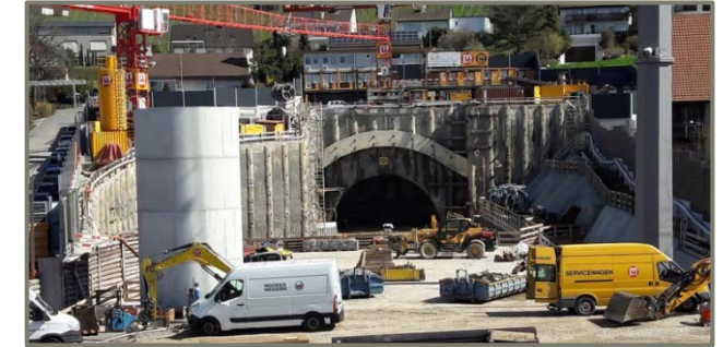
Driver portal side Weiningen
