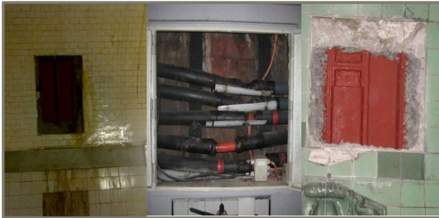
■ Deterioration of tunnel, utilities and steel segments
