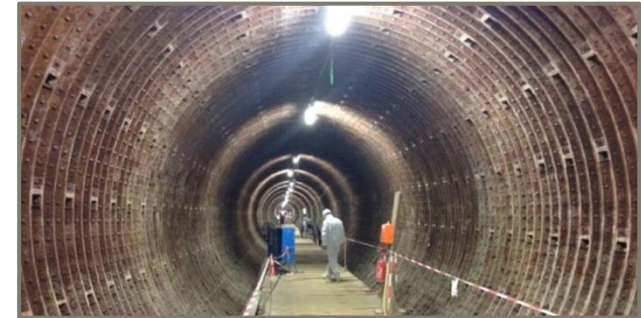
■ Corroded steel segments after concrete stripping
